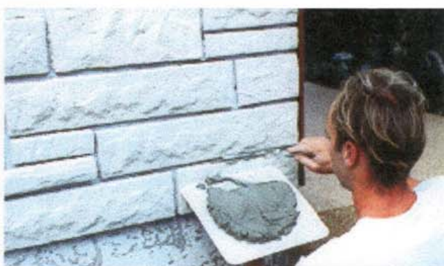
Space filling / grouting should be performed after some square meter work progress
